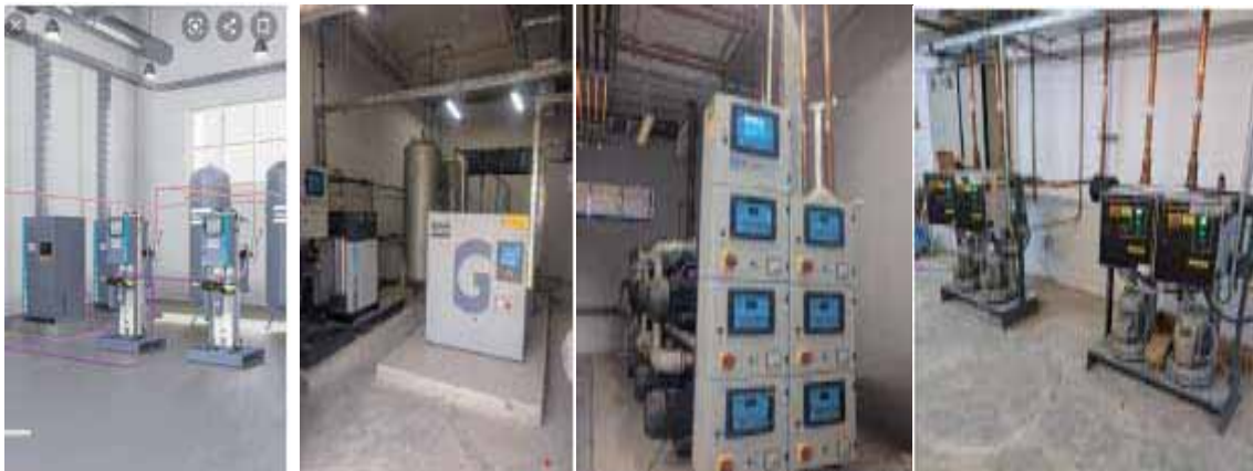
Medical gas delivery systems
